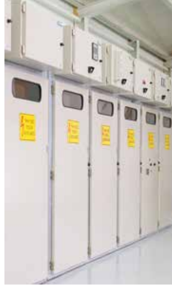
Medium-voltage switchgear system
