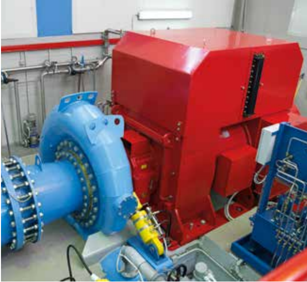
Francis turbine, synchronous generator, and hydraulic unit
