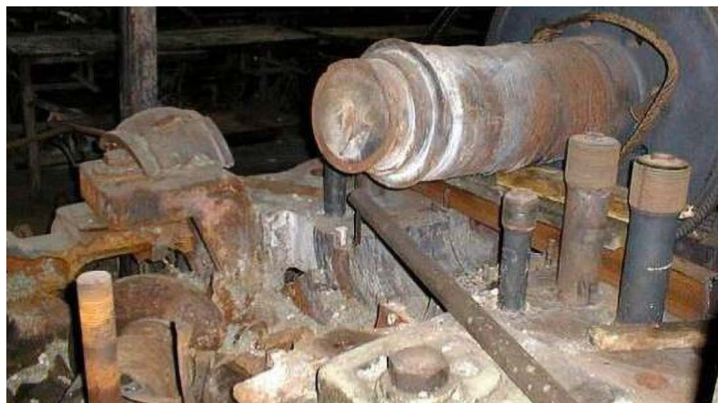
Modern protection features such as provided by Machinery Protection can reliably prevent this type of damage.
