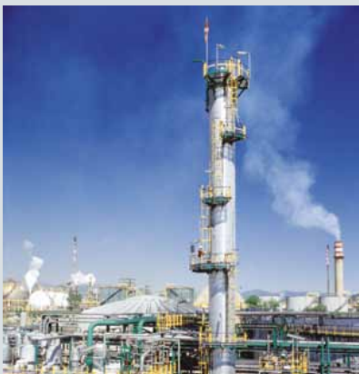
Zimpro® wet air oxidation system uses oxygen to treat high strength styrene monomer and polyol wastewater at Repsol YPF, Tarragona, Spain.
