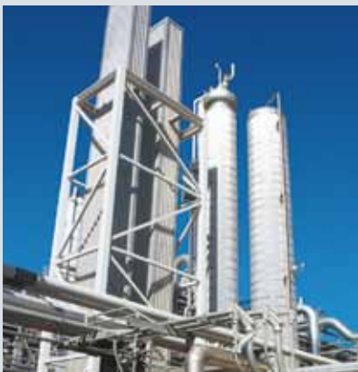
Zimpro® wet air oxidation system treats the spent caustic effluent generated by the world's largest naphtha steam cracker at the BASF ethylene facility, Port Arthur, Texas.
