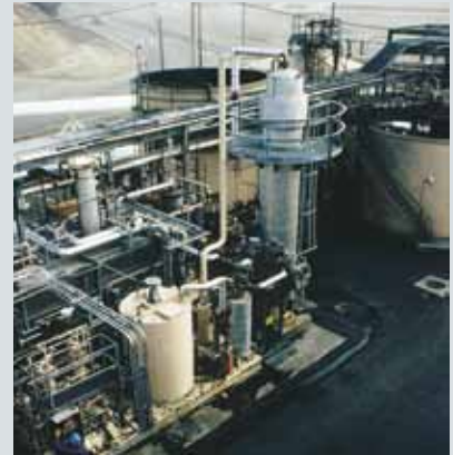
The wet air oxidation process is used to destroy biological solids and regenerate carbon at a Tosco refinery. In this application, the wet air oxidation process is referred to as the wet air regeneration process.
